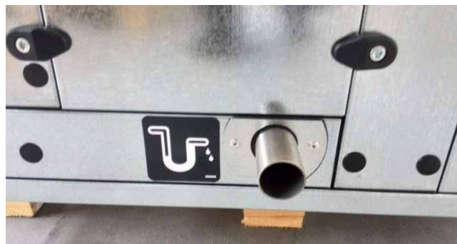
Condensate drain for the cooler (water/evaporator)
