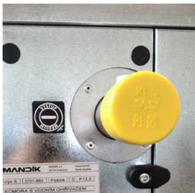
Marking of exchanger inlet
